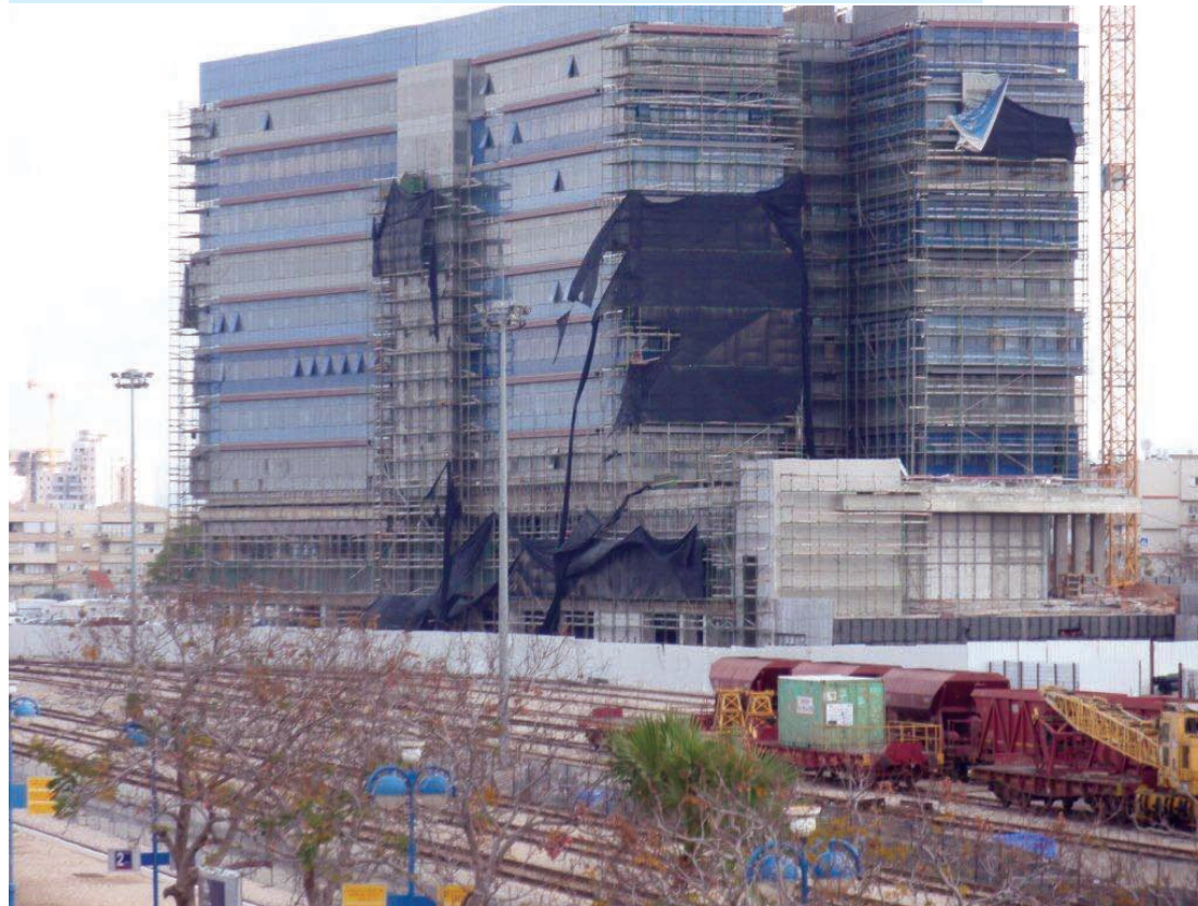
112:03 The new Israel Railways headquarters building takes shape at Lod station. (Photo 11.02.2016, Aharon Gazit.)
