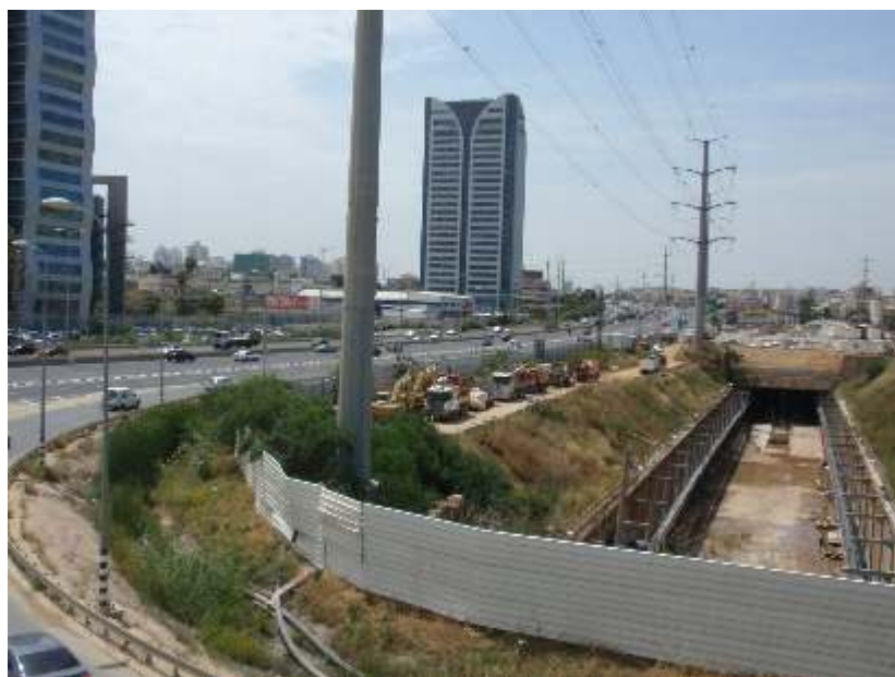
• View southwards towards B'nei Beraq and the future Em-HaMoshavot station (in tunnel); to Left the Petach Tikva high-tech area. Behind the photographer will be the depot at Kiryat Arie, Petach Tikva. (Photo: Aharon Gazit on 27.04.2018.)
