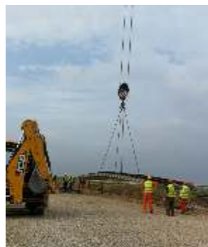
• Trackworks under way at km. 35 between Binyamina and Zikhron Ya'akov in April 2018. (Photos courtesy of IR Spokesman Israel Tal & Asst. Spokesman Matan Berkovich)
