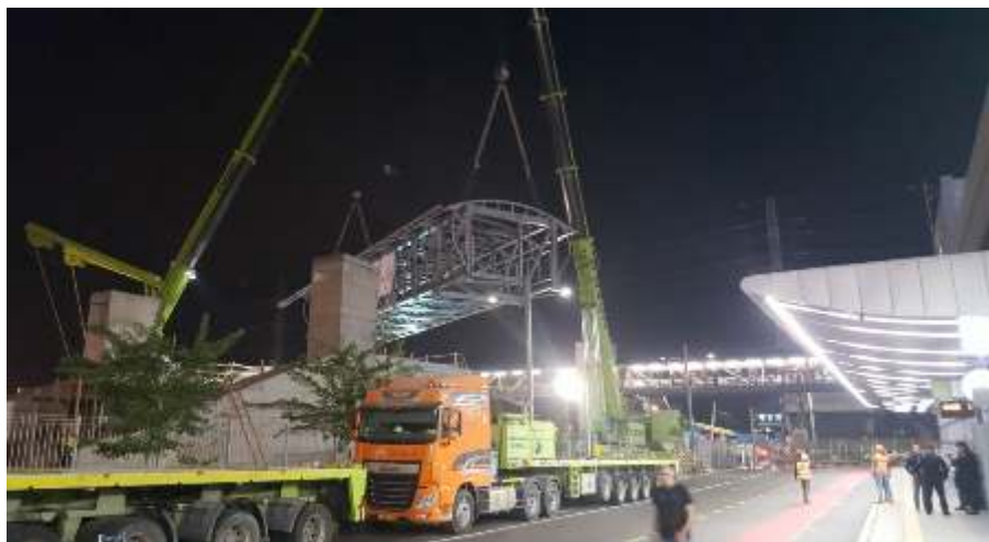
• The new bridge being installed. Photo courtesy of Matan Berkovich, IR press office.
