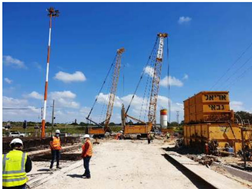
• Work on replacing a level crossing with an underpass. April 2020. (Photos courtesy of M. Berkovich.)
