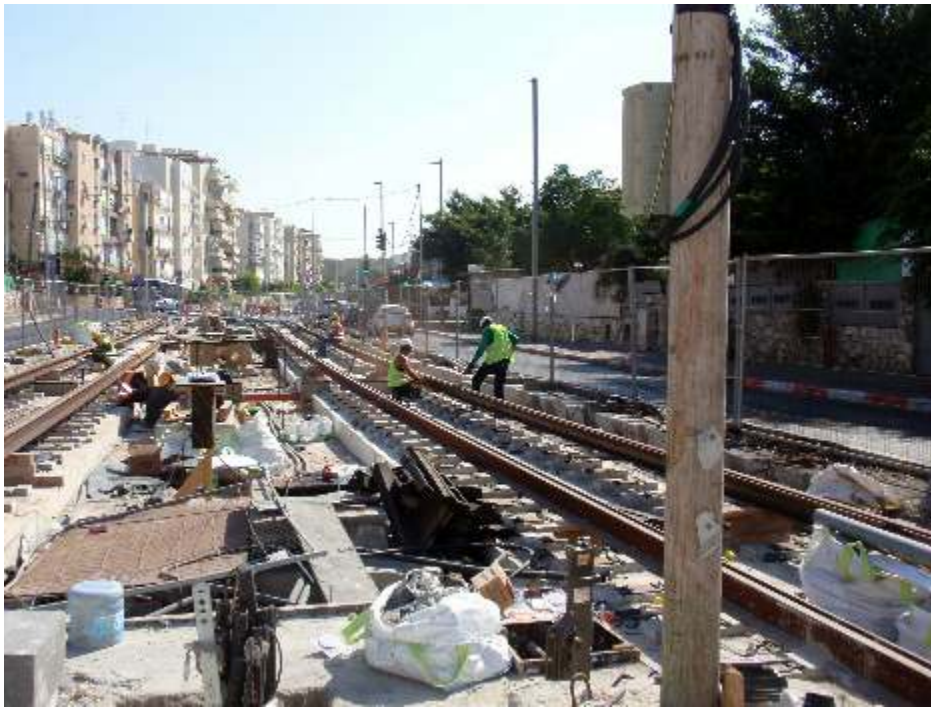
• Track works on the Tel-Aviv LRV/METRO Red Line at the city of Bat-Yam on various sections, taken on 18.10.2010 by Aharon Gazit-
