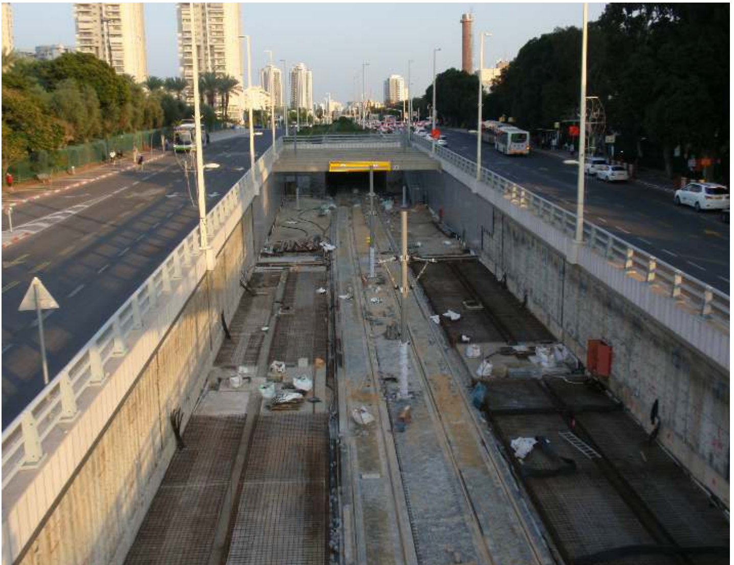
• Trackworks near the Beilinson Station (serving the Beilinson Medical Centre and the Avnat shopping mall) as at 01.12.2020. (Aharon Gazit) See also next page.....
