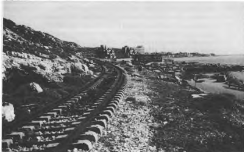
33:8. Former HBT track between Jubail and Bartroun. 31/3/96. Flat-bottomed rail on concrete sleeper with steel spacers - disused. (Photo: Andy Wilson).
