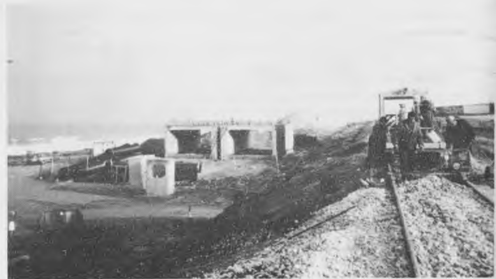
33:25: Carmel Beach, Haifa; Saturday 2/3/96. Precast concrete bridge units ready to be put in place on the following weekend, as a track machine works on ballast on the I.R. main line - work is in progress on doubling the tracks
