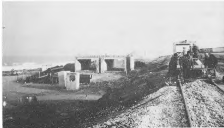
33:25: Carmel Beach, Haifa; Saturday 2/3/96. Precast concrete bridge units ready to be put in place on the following weekend, as a track machine works on ballast on the I.R. main line - work is in progress on doubling the tracks.
