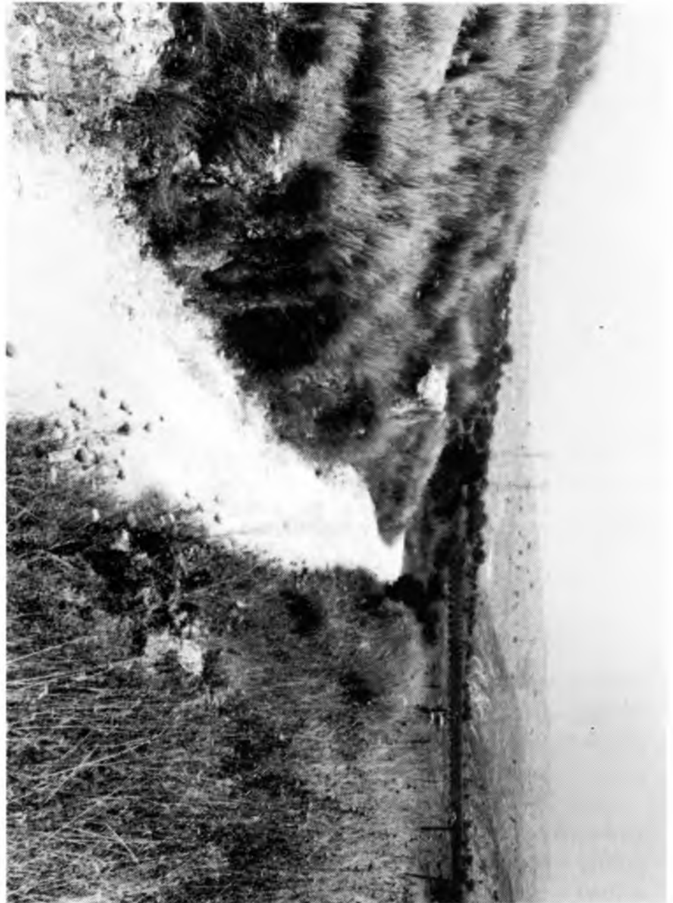
The cutting and crumbling stone retaining wall just short of the end of the standard-gauge track formation.
