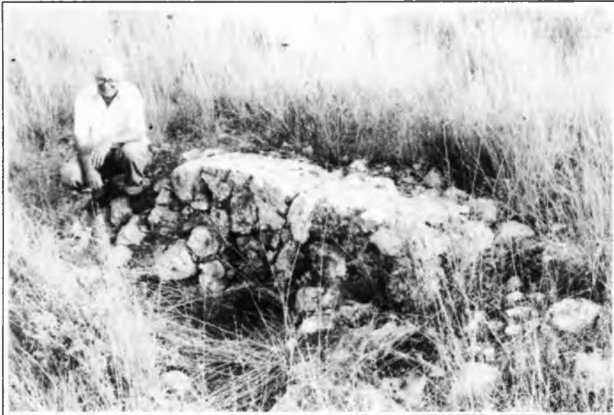
Photo 2: Uri Yinon inspects the decaying stone culvert built around a metal pipe
