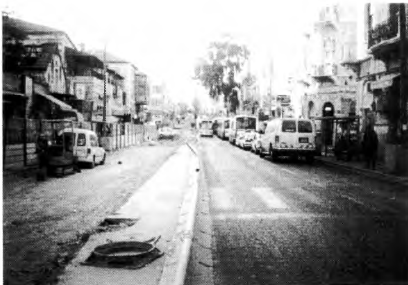
(Jaffa Road in Jerusalem - Works in connection with the Light Railway Project.)
