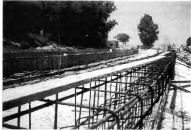
(Photos: below all by Sybil Ehrlich ) 3: Beit Shemesh Station under re-construction 26/07/02. 4: Beit Shemesh Station. 02/08/02. 5: Site of Jerusalem Zoo station. 13/08/02. )
