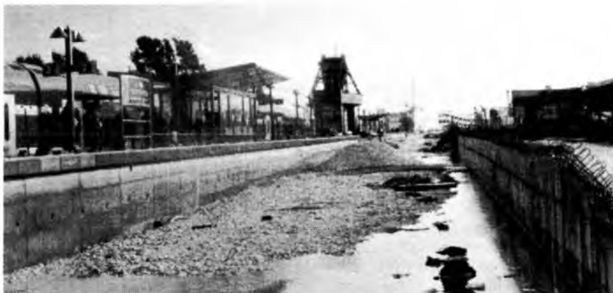
Ashdod Ab Halom - on the right the station building, at the left the new platform in use, at centre the new platforms and other buildings under construction.
