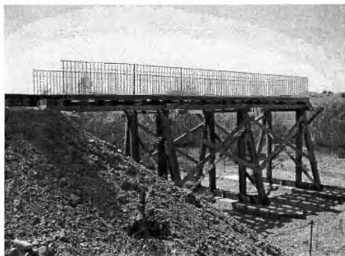
4. The new replica trestle bridge over part of Wadi Shellal built on the original concrete piers, seen in March 2004. (Photo: Erez Shalev.)
