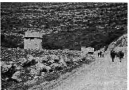
Photos show re-building work on the Jerusalem line near Bar Giora. Per Sybil Ehrlich.
