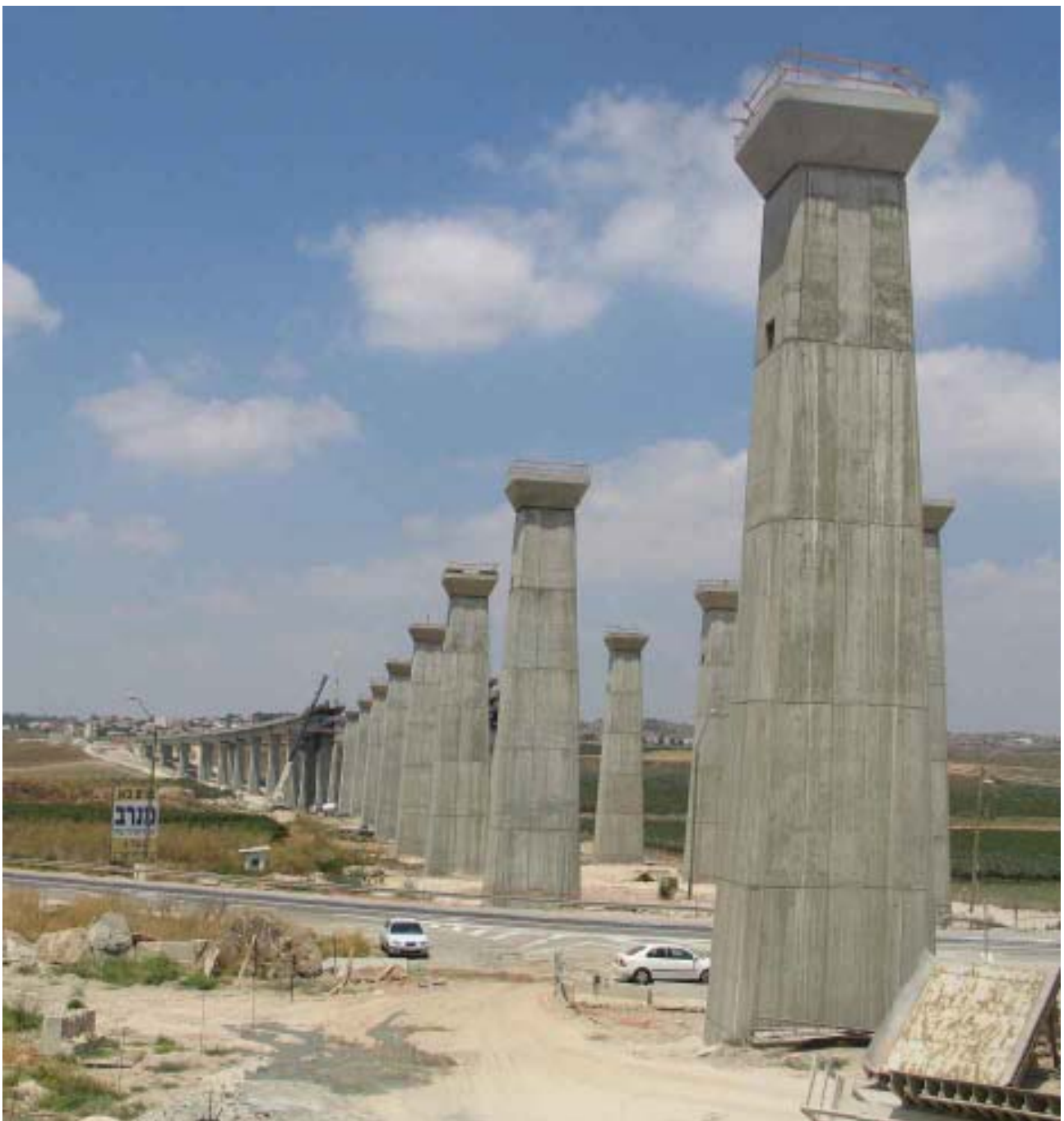
78:01. For once, not a train in sight - but the pillars reaching upwards to the heavens have an almost Classical effect; Or is it a Temple under way? A viaduct on the line to Jerusalem under construction. Photo by Jeremy Topaz.
